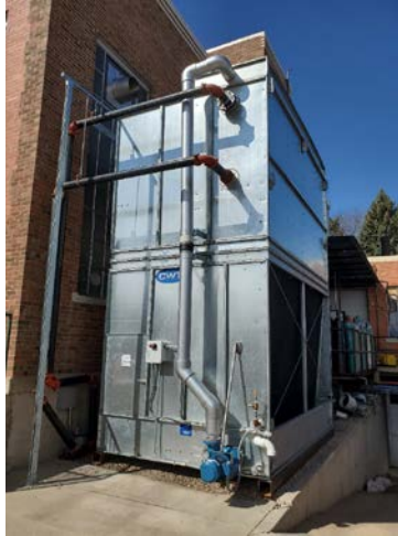
Figure 4-5 Condenser loop cooling tower
