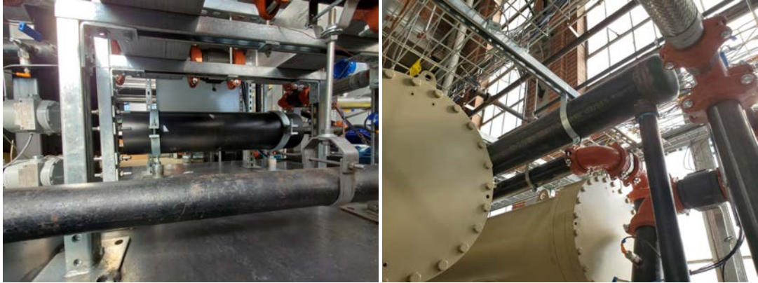
Figure B-4 Test facility accumulator (Left) and liquid receiver (Right)
