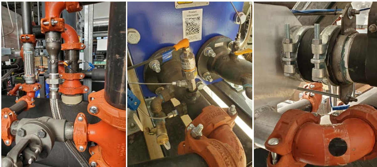
Figure B-18 Coupling strategies implemented throughout the test facility
