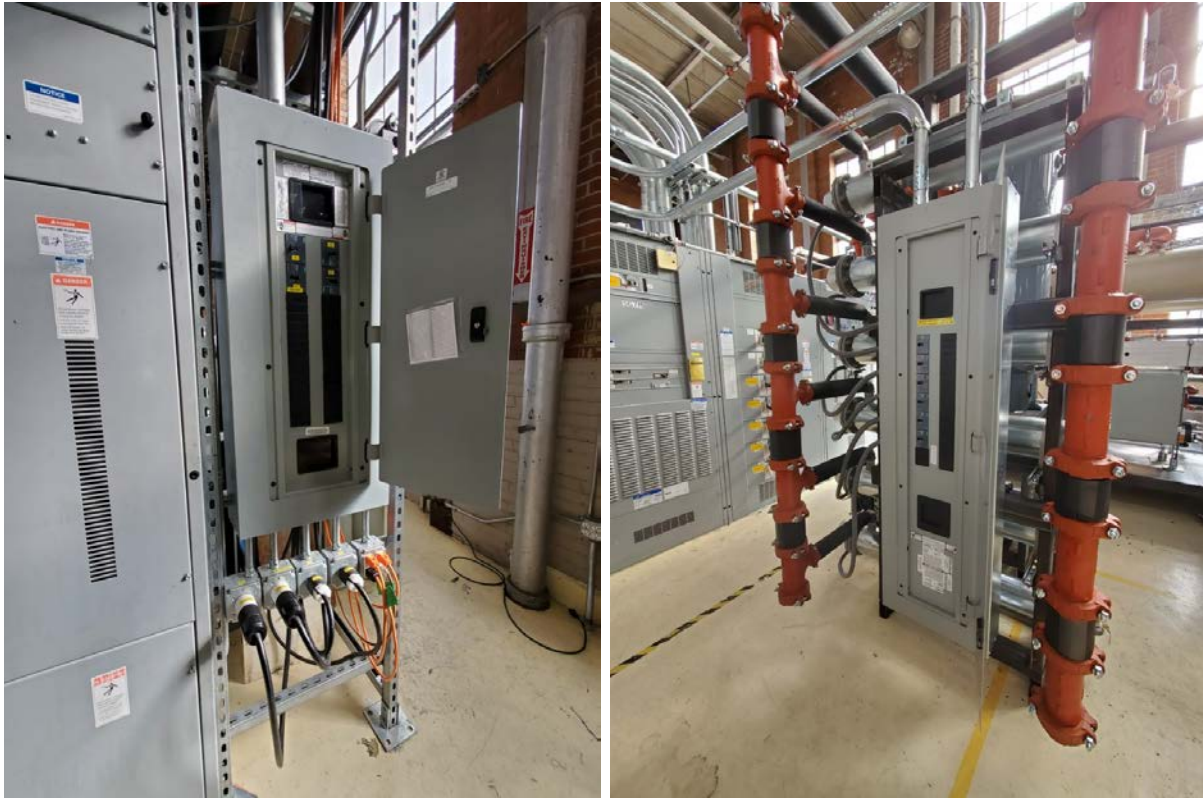
Figure B-7 Test facility electrical supplies
