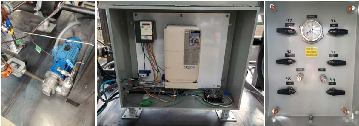
Figure B-2 (Left to Right) Fluid management pump, variable frequency drives, and fill/drain station
